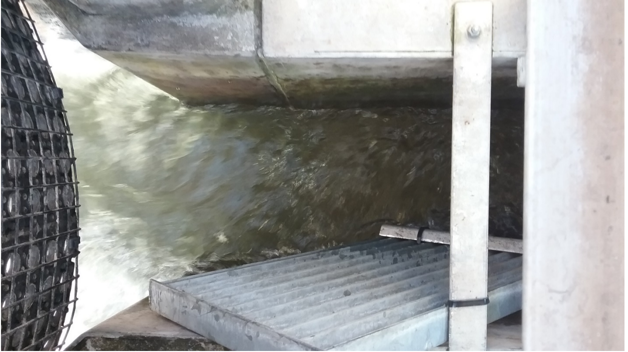
Photo 1. Looking down on failed false weir grating.
